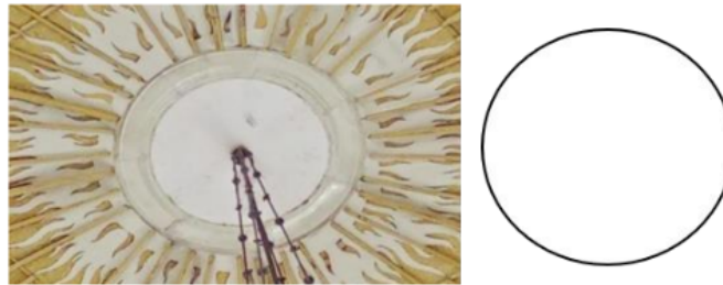
Figure 5. Yellow dome building void
