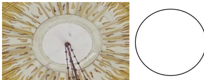
Figure 5. Yellow dome building void
